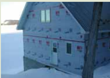
A weather barrier applied to the exterior sheathing prior to siding materials, acts as an additional barrier against wind, rain and snow.
